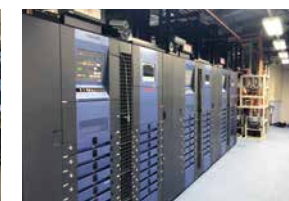
Transmission Station in Tokyo Sky Tree
