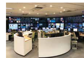
Network Control Center
